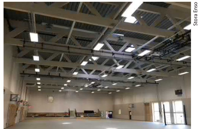
Figure 2.81. LVL roof trusses. Ydalir, France.
